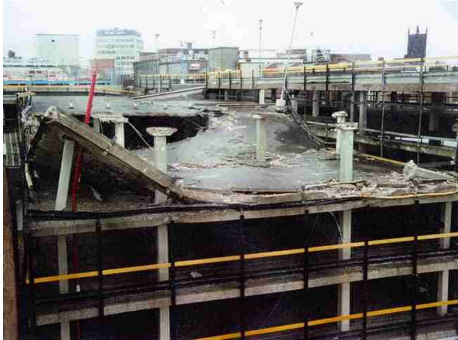
Figure 9.4. Pipers Row Car Park, Wolverhampton, England, progressively collapsed under its own weight. (Photo by courtesy of the HSE, UK).
