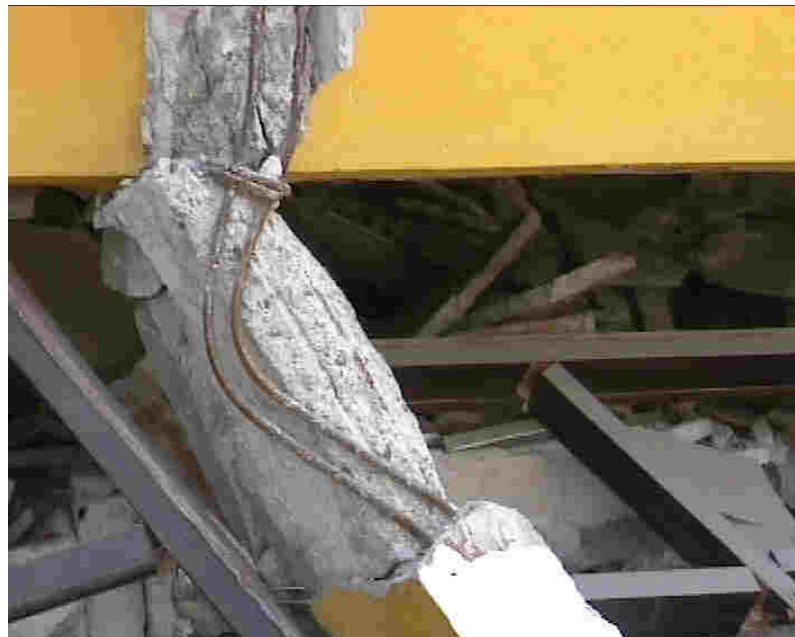
Figure 9.2: Failure due to poor quality design and/or construction – the absence of stirrups in the column. (Photo by courtesy of EEFIT, 1999)
