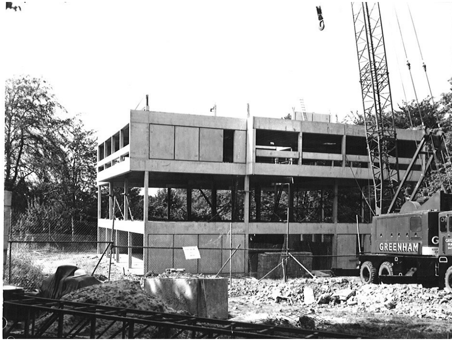
Figure 9.1 Aldershot building prior to the collapse (Photo: UK Crown Copyright.)
