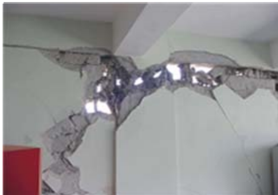
Column end failure
