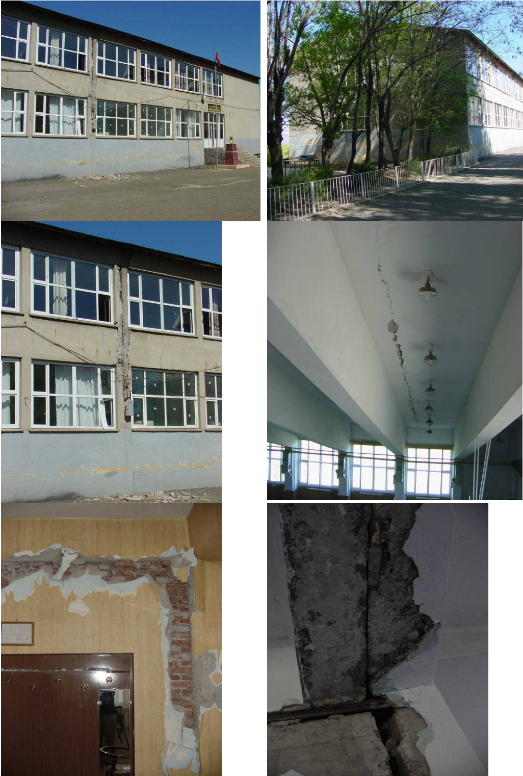
Figure 6. Anadolu Ogretmen High School after 2003 Bingol Earthquake (Moderate)
