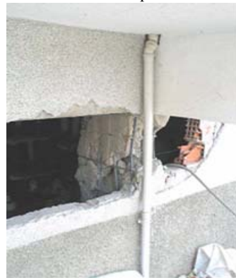
Shear failure of short column
