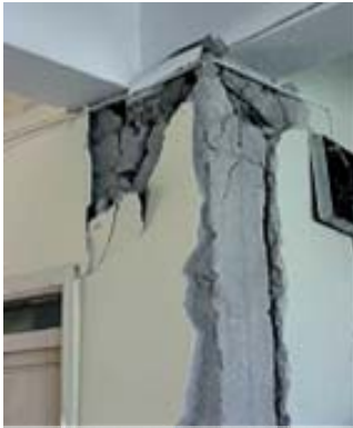
Column and beam damage
