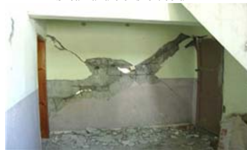
Shear walls failure
