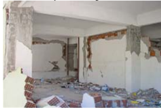
Spalling and crushing concrete due to high axial loads
