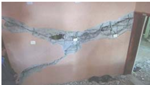
Shear failure of shear walls (at ground and first floor)
