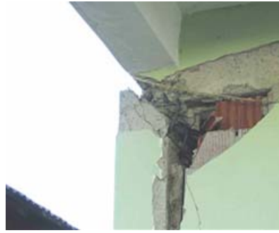
Separation of column due to improper detailing
