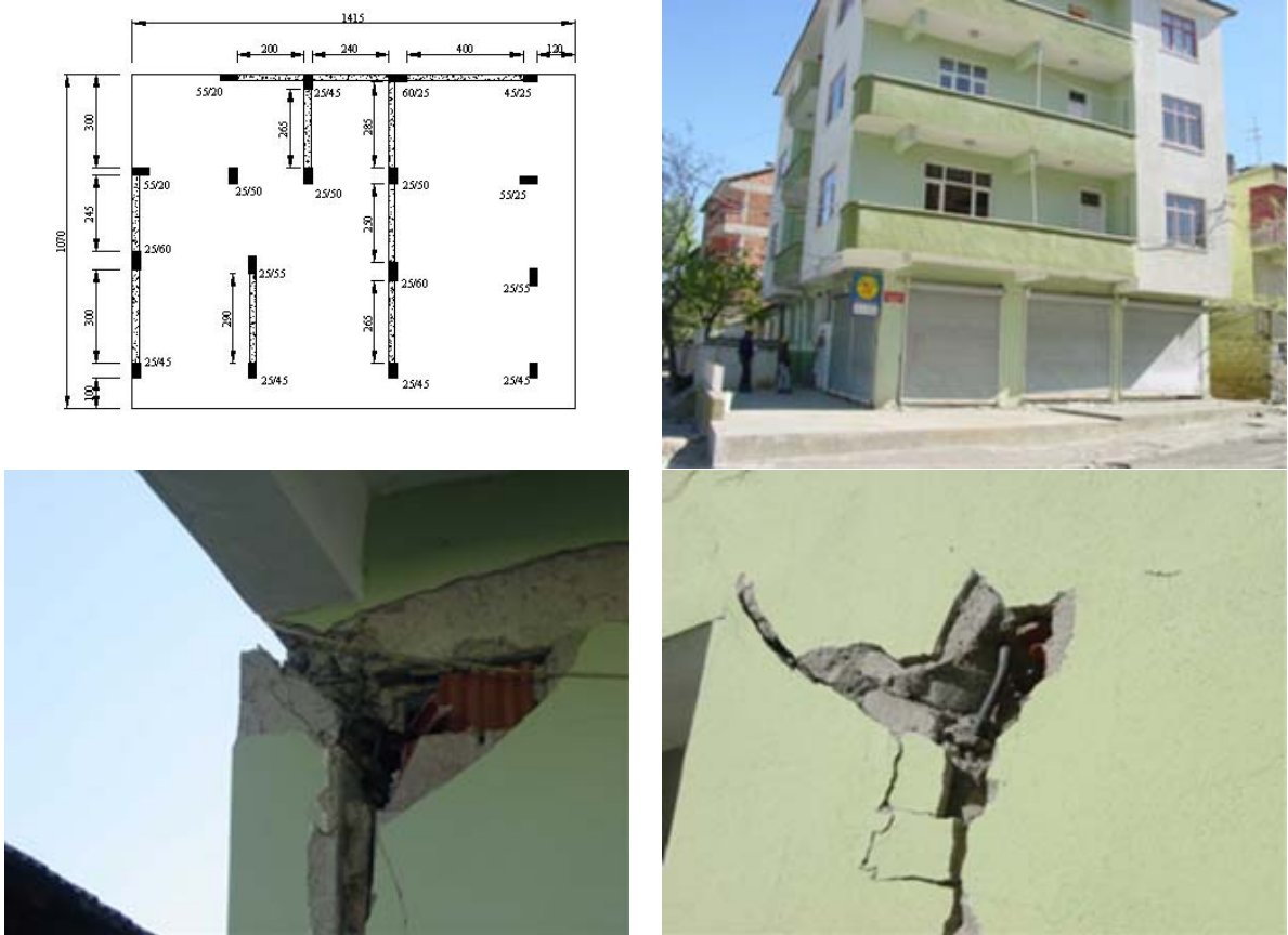
Figure 10. Typical residential building after Bingol Earthquake (BNG-11-4-2)
