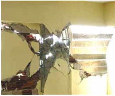
Brittle failure of column and buckling of bars
