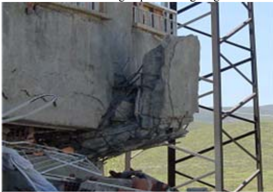
Insufficient confined column
