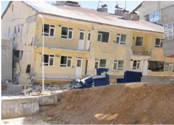
Ground story collapse of 3-story building
