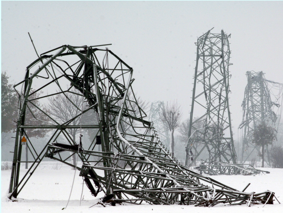
domino-type collapse of overhead transmission line towers triggered by ice accretion (Germany, 2005)
