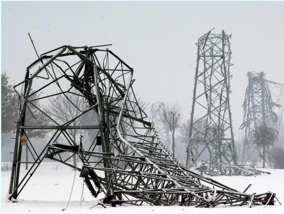
domino-type collapse of overhead transmission line towers triggered by ice accretion (Germany, 2005)
