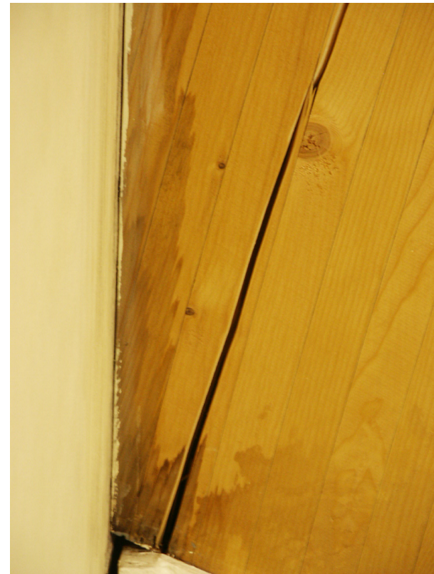
Crack in glulam arch Typically low consequence
